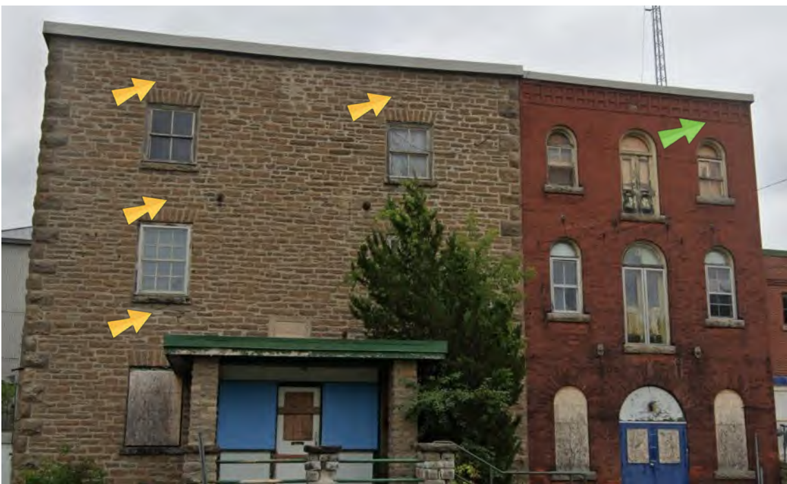
Fig 10. Note that mortar cracks at RE2, 3E2, 2E2, and RE4 existed before the fire.
