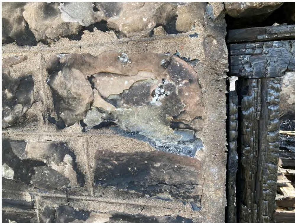
3A1 spalled out-of-bed sandstone Sample locn
