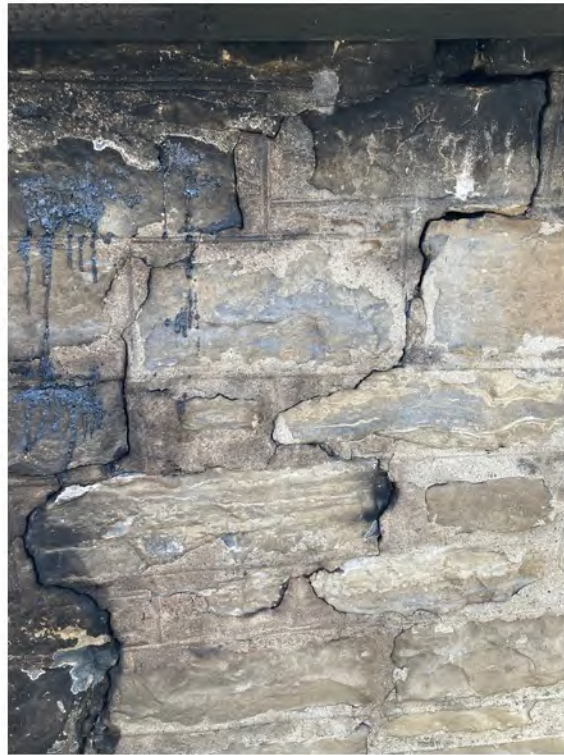
RE1 pyramidal crack
