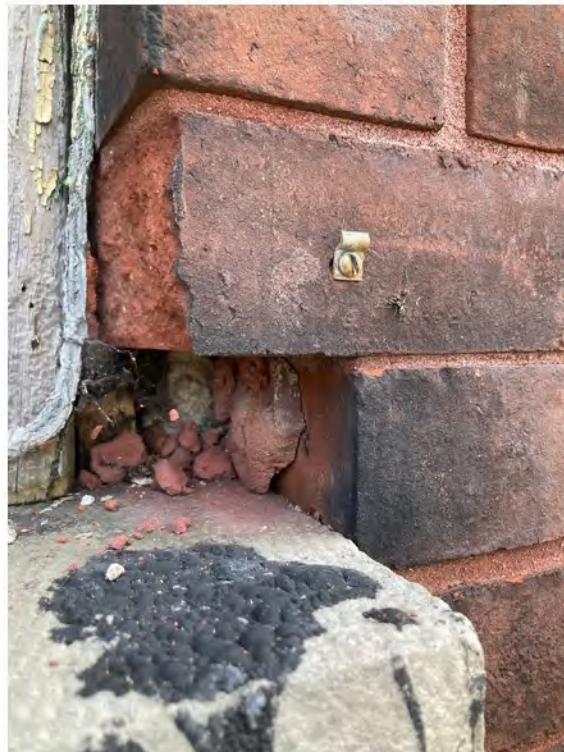
2E7 mortar sample locn
