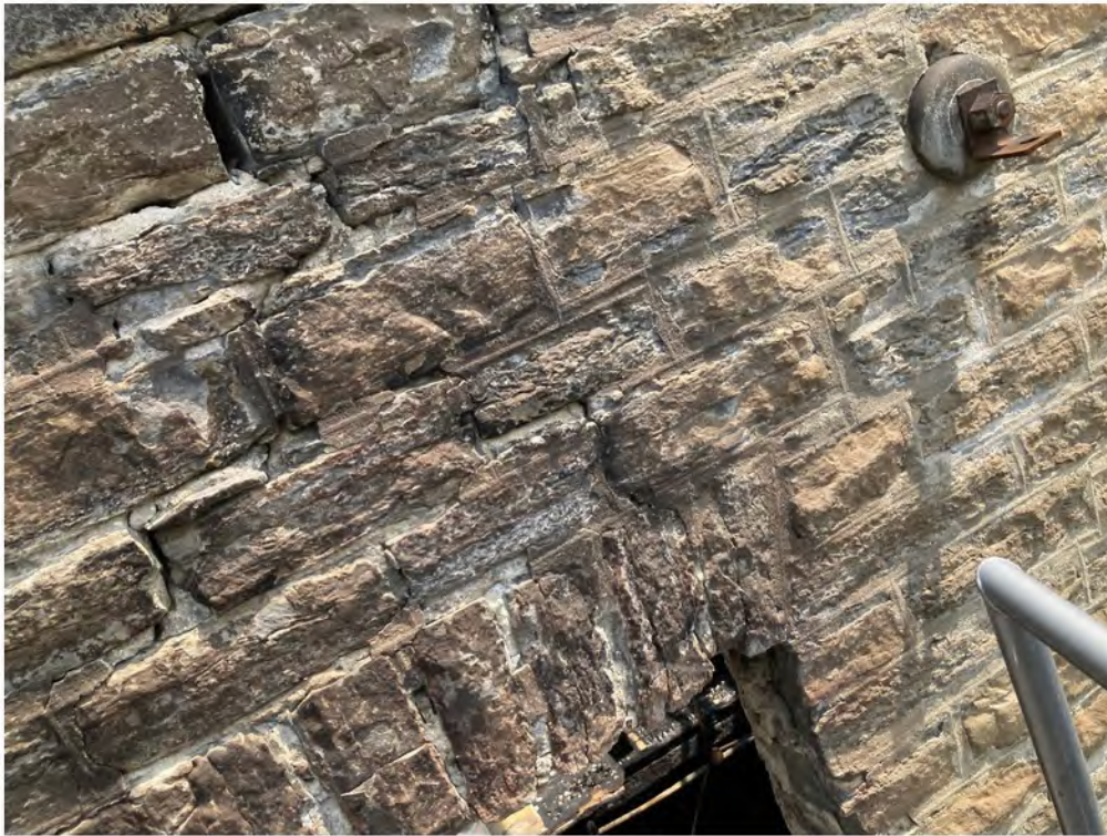
2E2 pyramidal cracking
