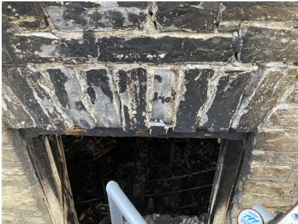
MB1 window voussoir Spalled lintel stone sample locn
