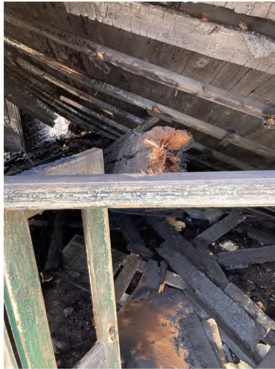
3E6.5 window frame supporting failed roof beam
