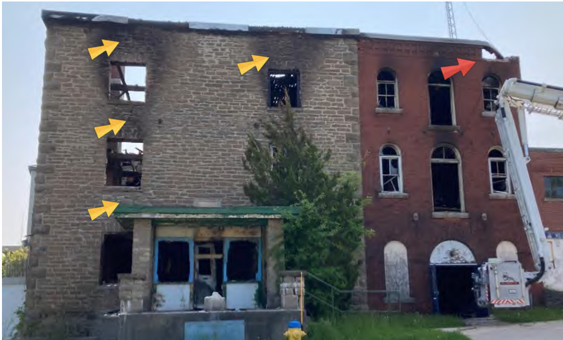
Fig 9. Note the appearance of post-fire cracks at RE2, 3E2, RE4 and parapet damage at RE8.
