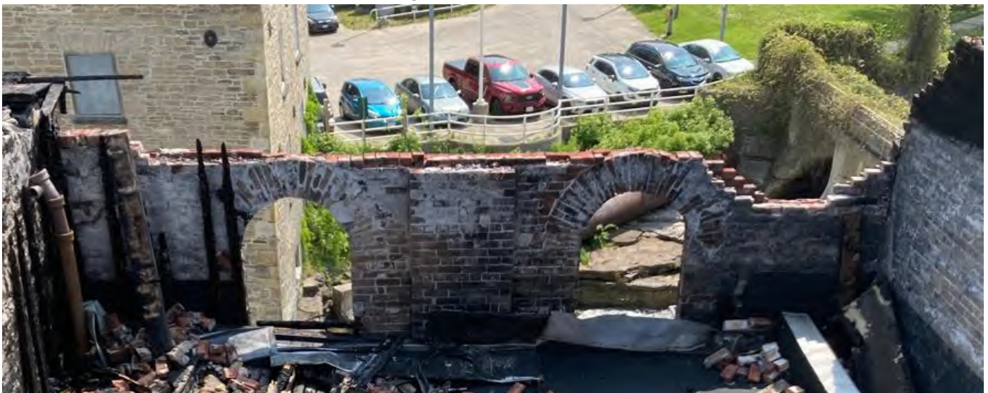
Fig 19. View of Building 3 rear wall at 3 rd level along the roof line (RA5-RA8).
